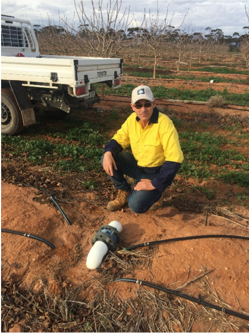
Figure 2. Andrew Bowring with a non-return valve brought to the surface on an uphill submain
